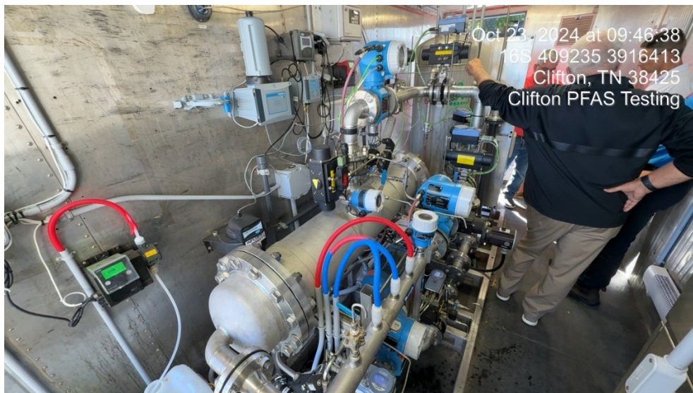
CUF On-Site Pilot; Full Remote/ Automation/ LT2 Compliant/ ANSI/CAN 61-372
